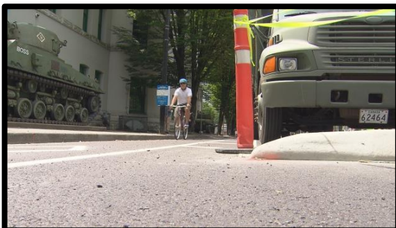
City crews began work last week, but the plan to upgrade the bike lane has been publicly discussed for years, including in city council and an open house, said Lon LaClaire, director of transportation for the City of Vancouver. (CBC)
