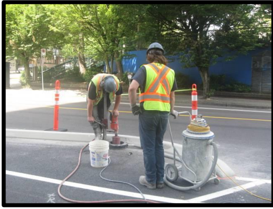
Workers are installing concrete barriers on the new bike lanes. Photo: Carlito Pablo
