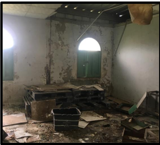
Heavily damaged school in Kodok
