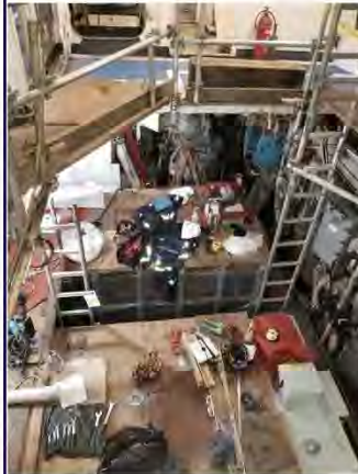
CAT 32 Diesel Installation in After Auxiliary Machinery Room
